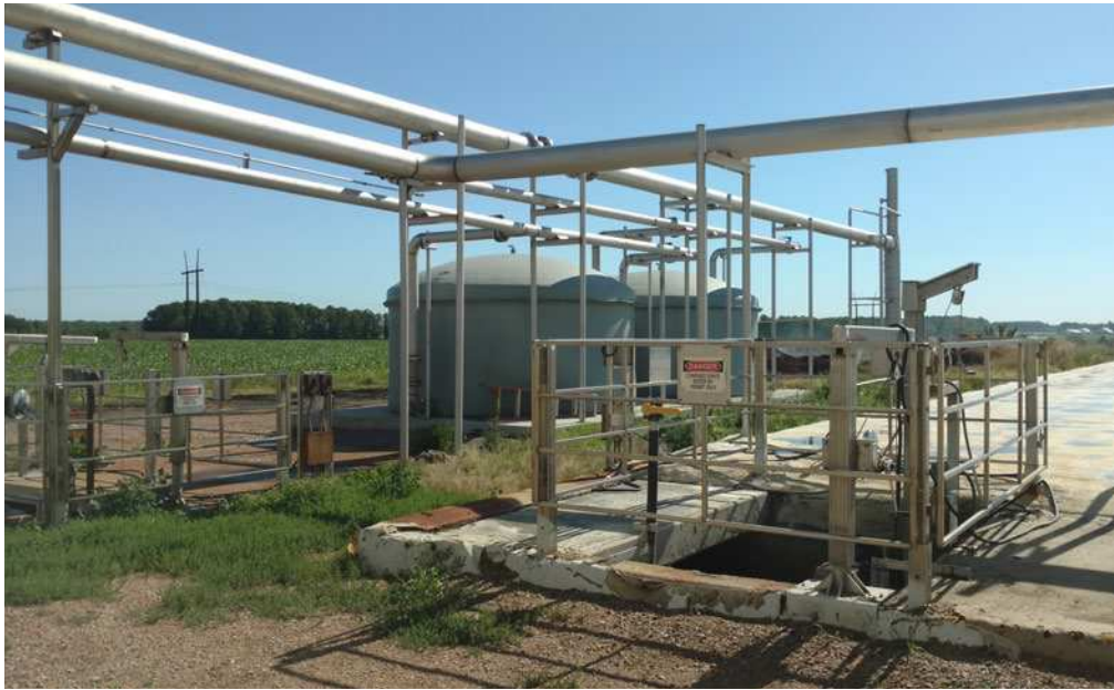
Norm-E-Lane's anaerobic digester and CHP system produce renewable power, along with a nutrient-rich byproduct used as fertilizer to grow crops.
