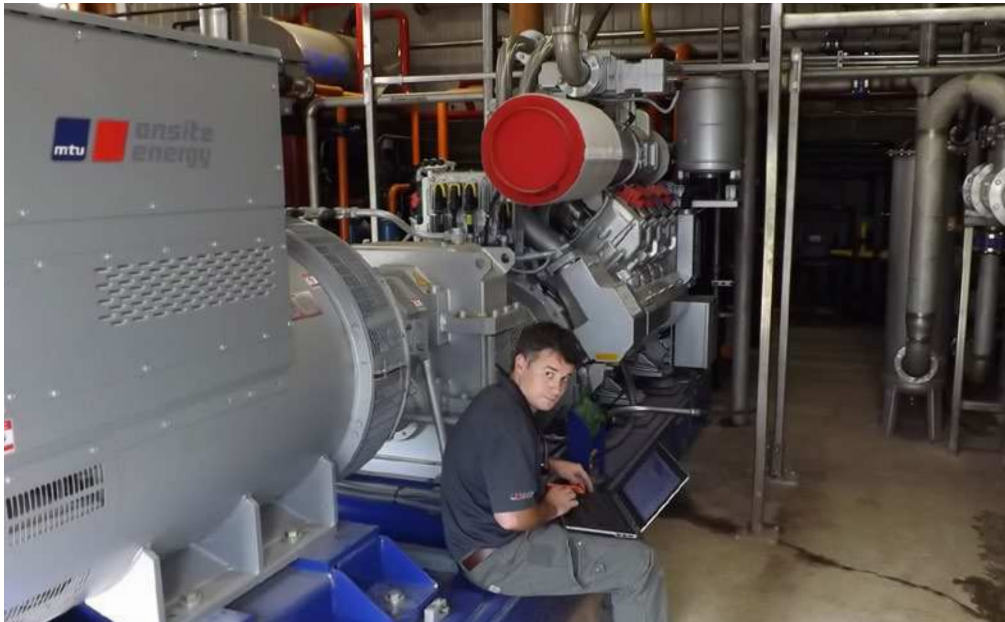
A service technician from W.W. Williams inspects the CHP system to ensure reliable continuous operation.
